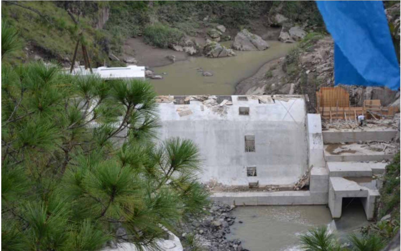
Construction of Corral de Piedras hydroelectric dam. Water was granted in concession to Energía de Occidente ENERCO company for 20 years.
