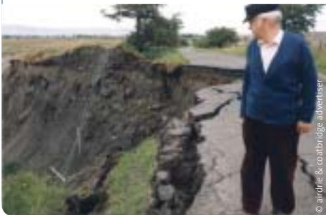
A public road used by school buses falls victim to the greed for more coal in Lanarkshire, Scotland.
